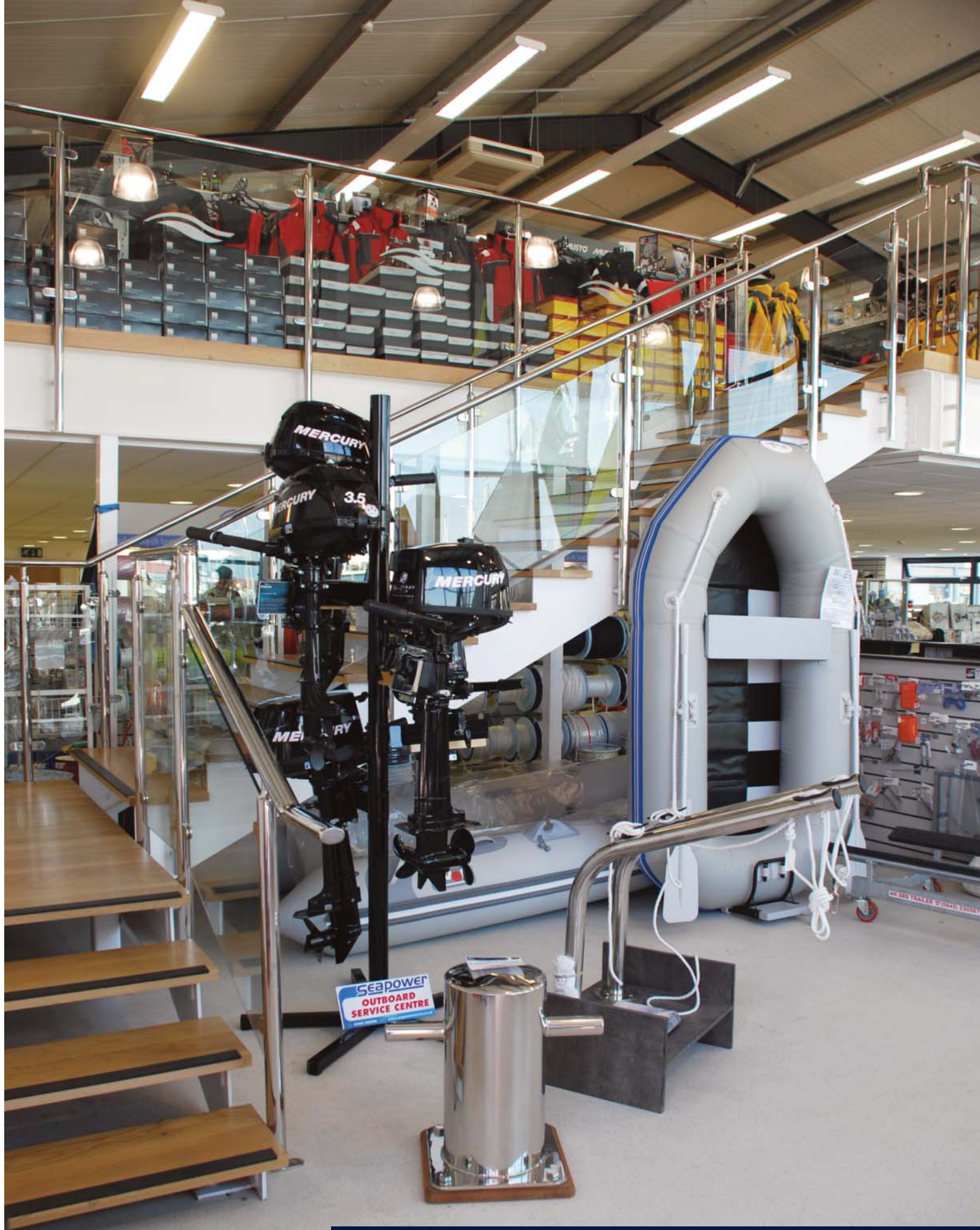
Glass balustrading in a commercial premises - 10mm toughened glass panels were installed using the customers stainless steel rails and clamps. Each parallelogram was templated to ensure panels fitted correctly.
